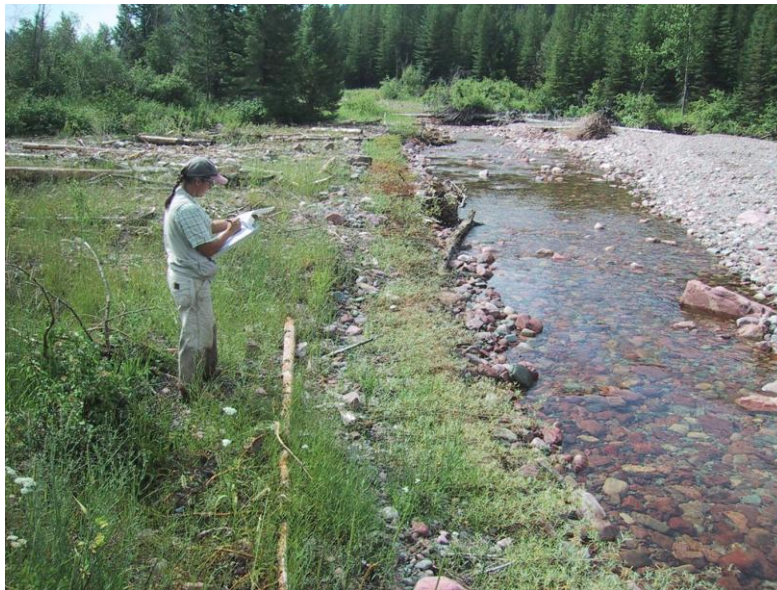
Photo 7: Dunham Creek Photopoint 1 at the upstream end of the project, looking downstream. The bank treatment here is a coconut-fiber soil lift, layered with willow whips above and below the wrap. A planting pod is installed in the floodplain to the left.
