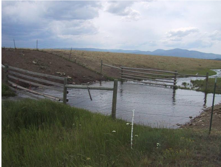
Photo 30: View of property downstream of the Middle Rock Creek project. No riparian enclosure exists on that portion of the stream, and the stream channel is markedly wider than on the project area.
