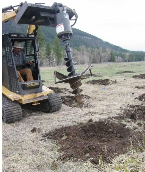
Photo 32: Augering holes for T1 size plants using a tracked skidsteer mounted with a two-stage scalping auger, resulting in a 9” wide by 18” deep hole plus a 36” sod scalp.
